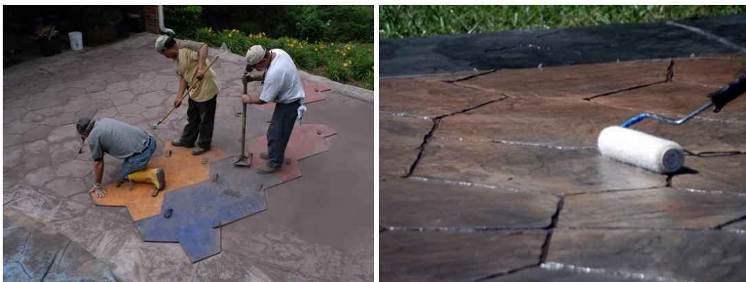
Figure 9: Stamps being used to imprint fresh concrete, and sealer being applied in the final stage (Concrete Network 2019)
