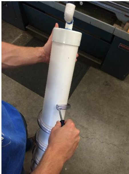
Figure 5-9 a screw being tightened on the Archimedes Screw Pump
