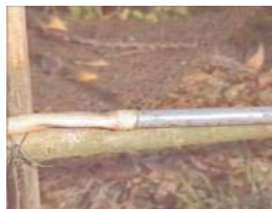
Photo 48. Connecting a plastic hose to the PVC pipe of the gas outlet
