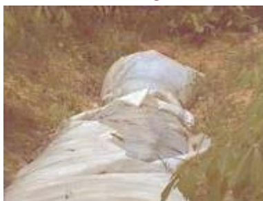
Photo 81. The outer plastic layer damaged (after 3 years..!). The inner one is still gas-tight.
