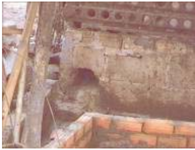
Photo 64. A channel is made with bricks to lead the waste from the pig pen to the inlet of the biodigester
