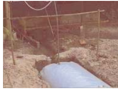
Photo 65. The channel is connected to the biodigester
