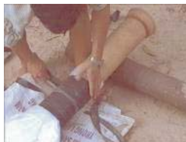
Photo 23. Wrapping the rubber bands around plastic tube where it overlaps the pipe
