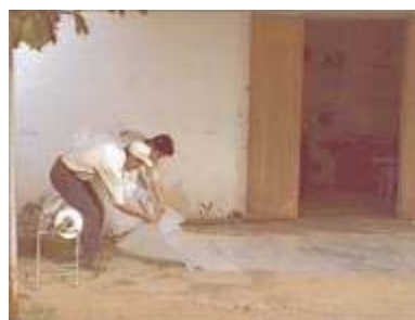
Photo 9. Starting to put one plastic tube inside the other to give added strength
