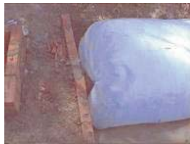
Photo 89. A small wall of brick to avoid the soil entering and rain water entering the biogas digester.
