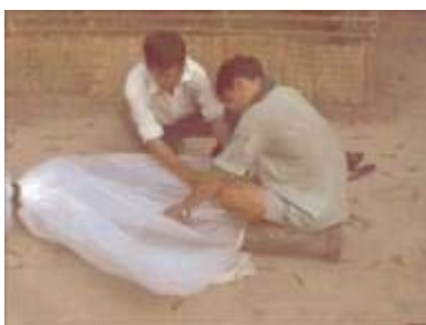
Photo 31. Placing the outlet pipe (following the same procedure as for the inlet pipe)
