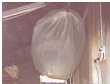
Photo 59. The reservoir bag full of biogas
