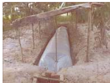
Photo 69. Roofing can protect the biogas digester
