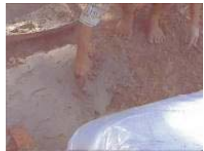
Photo 90. A mixture of soil and cement to cover upper part of the walls of the trench
