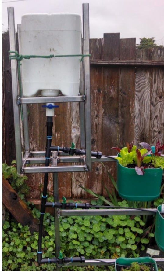
Figure 5-5: The reservoir tank dispenses water to the main 1/2 inch tubing line of the irrigation system.
