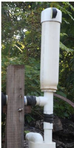
Surge chamber on a rower pump: 4" Sch 40 PVC, 18" long
