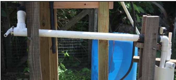
Rower pump installed at a borehole
