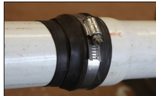
The foot valve joint, wrapped in rubber and hose clamped
