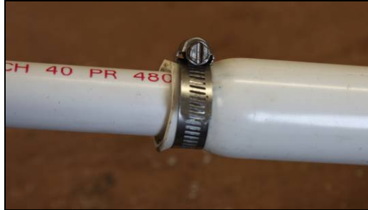
1.25" pipe compressed onto 3/4" pipe with hose clamp
