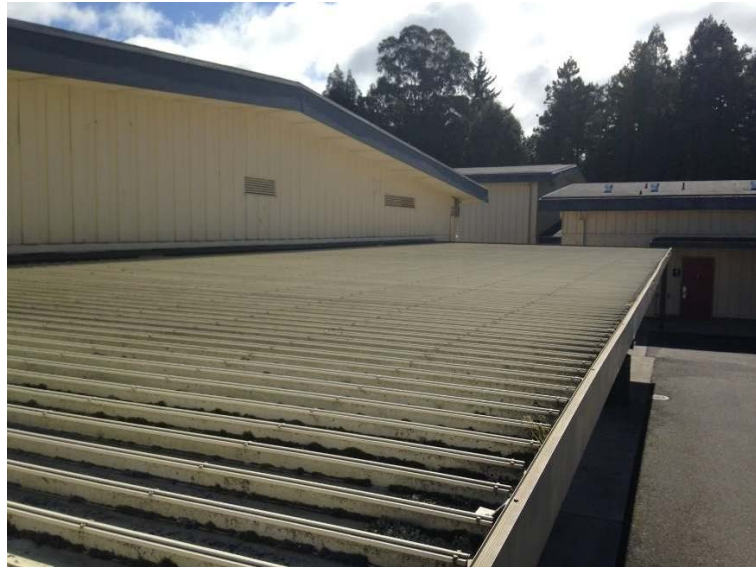
Figure 9: The picture shows one section of the awning roof and the gutter along the edge farthest from the wall of the adjacent building. It can be seen from the photo that the gutter opening is narrow. Picture taken by Ahron Cervania.
