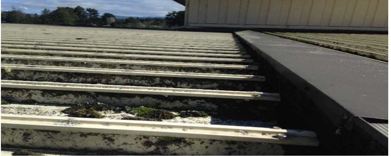
Figure 7: On the right of the figure between the grey metal and the silver sheet metal roofing, is the inaccessible gutter. The silver metal in the picture will be cut in order to increase access to the gutter. Picture by Ahron Cervania.
