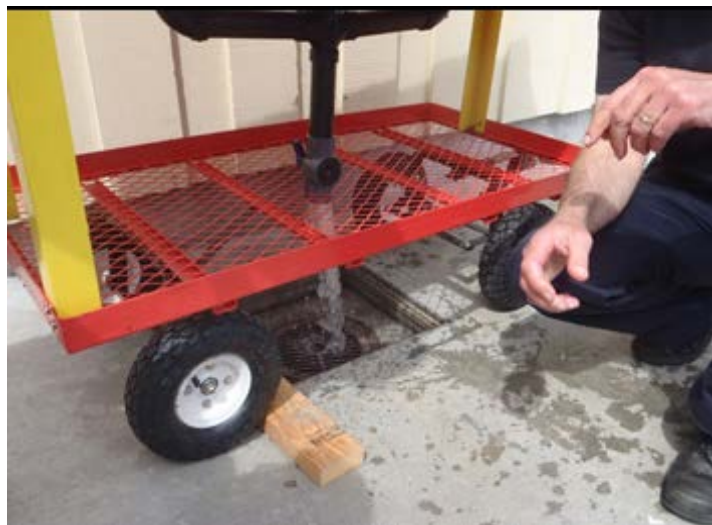
Figure 5.2.9: Shows the Acrylonitrile Butadiene Styrene drainage system releasing used water into the sewer drain.
