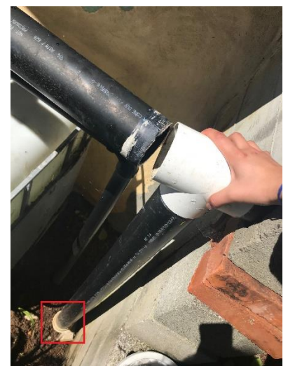
Figure C-2. Check the integrity of the cap shown in red
