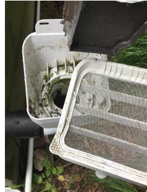
Figure C-1. Screen can be easily taken off to check the pipe underneath
