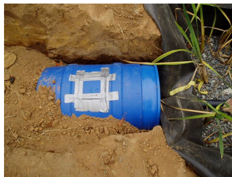
Figure 2-4: Surge tanks and marsh baffles (“CCAT greywater marsh” 2011)
