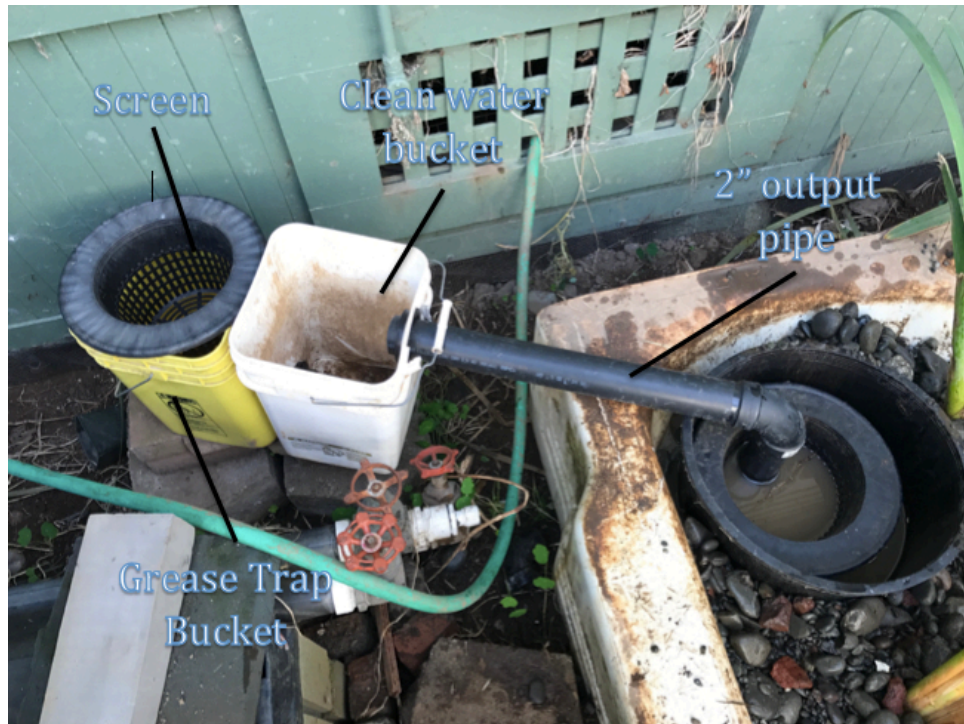
Figure 5-3: Input tank and grease trap, angle view, taken by Jennifer Turk on 12/2/16
