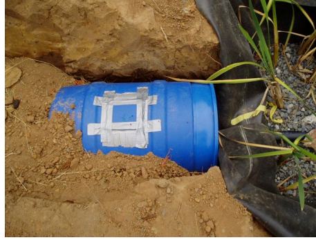
Figure 24: Surge tanks and marsh baffles (“CCAT greywater marsh” 2011)
