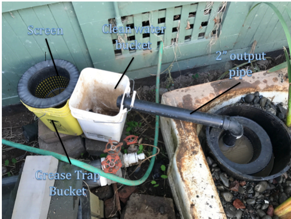
Figure 53: Input tank and grease trap, angle view, taken by Jennifer Turk on 12/2/16
