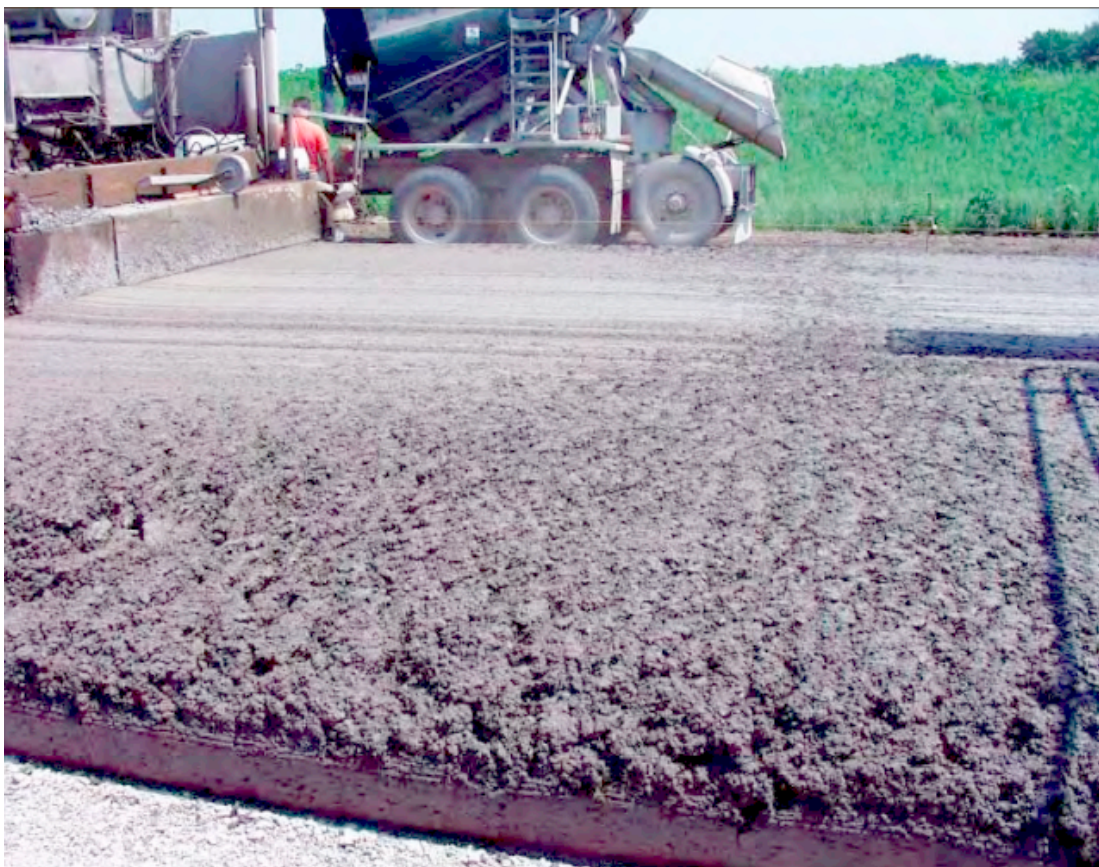
Figure 4: Segregation of Concrete (“Integrated Materials...”)
