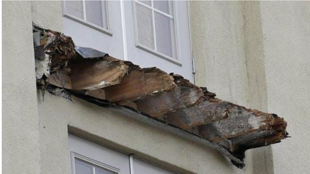
Figure 2.2.8.2: An example of dry rot in wood caused by fungal decay (Archinect.com).
