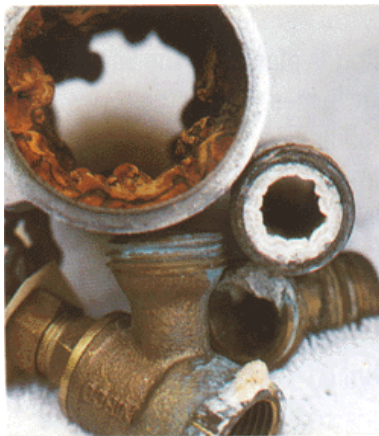
Figure 2-7: Pipe with deposits caused by hard water ( http://chemwiki.ucdavis.edu/@api/deki/files/1134 )
