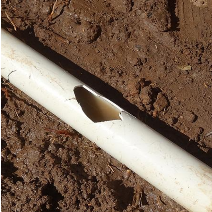
Figure 2-4: Broken PVC Pipe http://www.home-dzine.co.za/garden/garden-cracked-pool-pipe.htm
