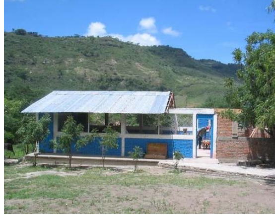
Figure 10. A school building under construction in a rural Nicaraguan community. (Photo from www.seadsoflearning.org )
